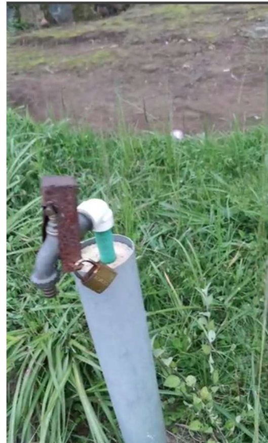
Alabukam Health Center – A public tap in front of the building (Needs repairs)
