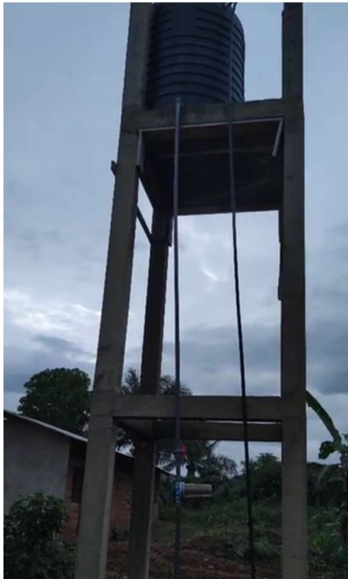
2000 L Tank at Alabukam Health Center
